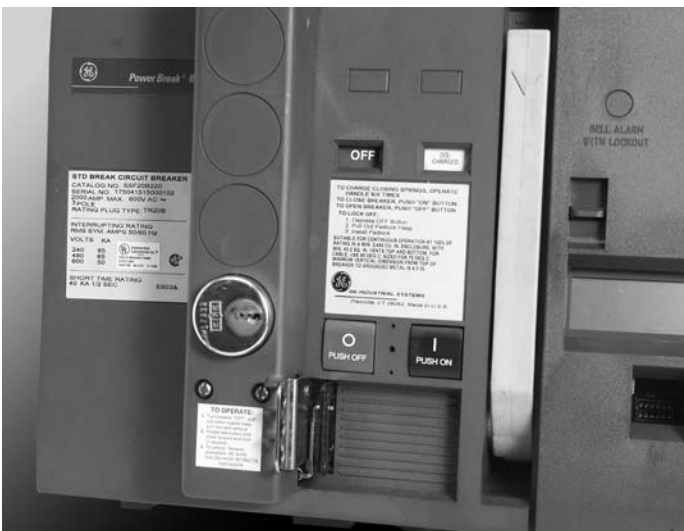
Key interlock installed on front of the breaker
