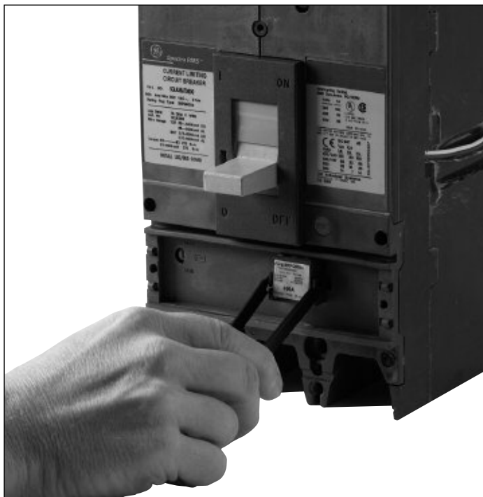
Fig. 6.1 Removal of rating plug
